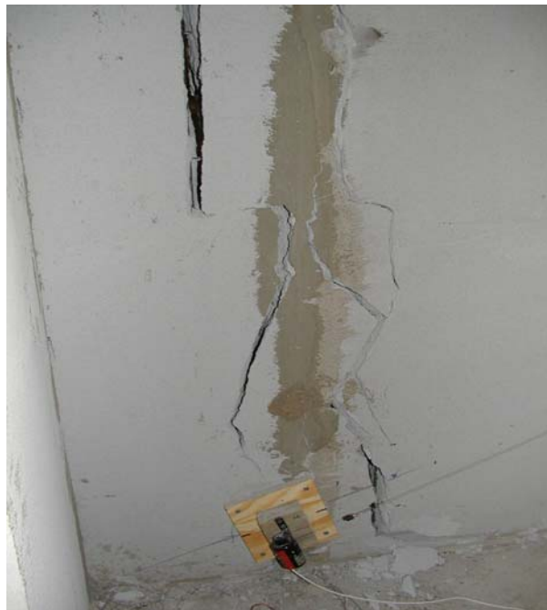
Figure 6.34 Vertical crack at the north end of east wall (base of first story wall)
