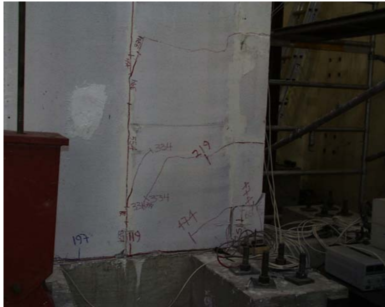
Figure 6.28 South compressive toe of Shear Wall specimen 15a at the end of the test
