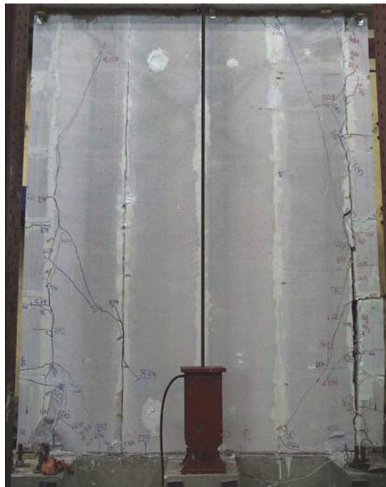
Figure 6.24 Vertical cracks at the north and south ends of Shear Wall Specimen 16 at the end of the test
